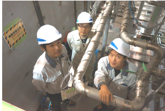
Fig.1 Heat Resistant FBG Sensor Installed at a Pipeline of the Sodium Loop under Construction at the TSURUGA SHIRAKI District. (2014 Oct. 31th)
