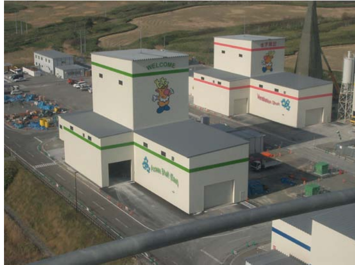
Figure 1.3: East Access Shaft (green highlighted building in the foreground) and the Ventilation Shaft (pink highlights in the background) are currently under construction
