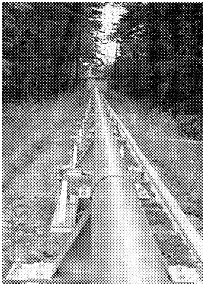
Photo 16.6 First one hundred meter part of 190 m neutron flight tube. The neutron detector station seen at the end of the tube is the 100 m one.
