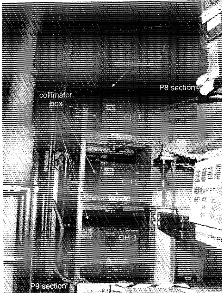
Figure 2.15. Photo of the Sci-Fi detector system on JT-60U.
