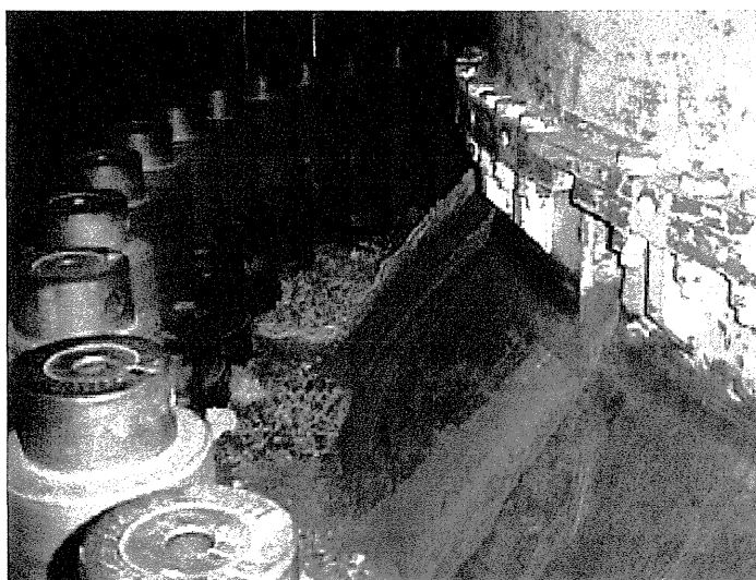
Figure 3-1 Boric Acid and Iron Oxide on Vessel Flange (11)
