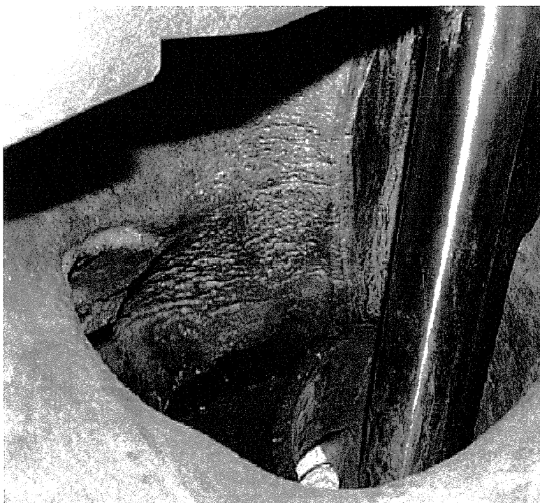
Figure 3-4 Cavity in Reactor Vessel Head Between Nozzle 3 and 11 (13)
