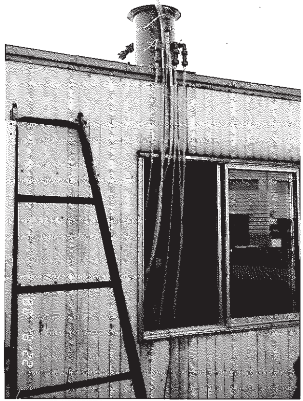
写 - 2 Hose Arrangement and Gravity Tank
